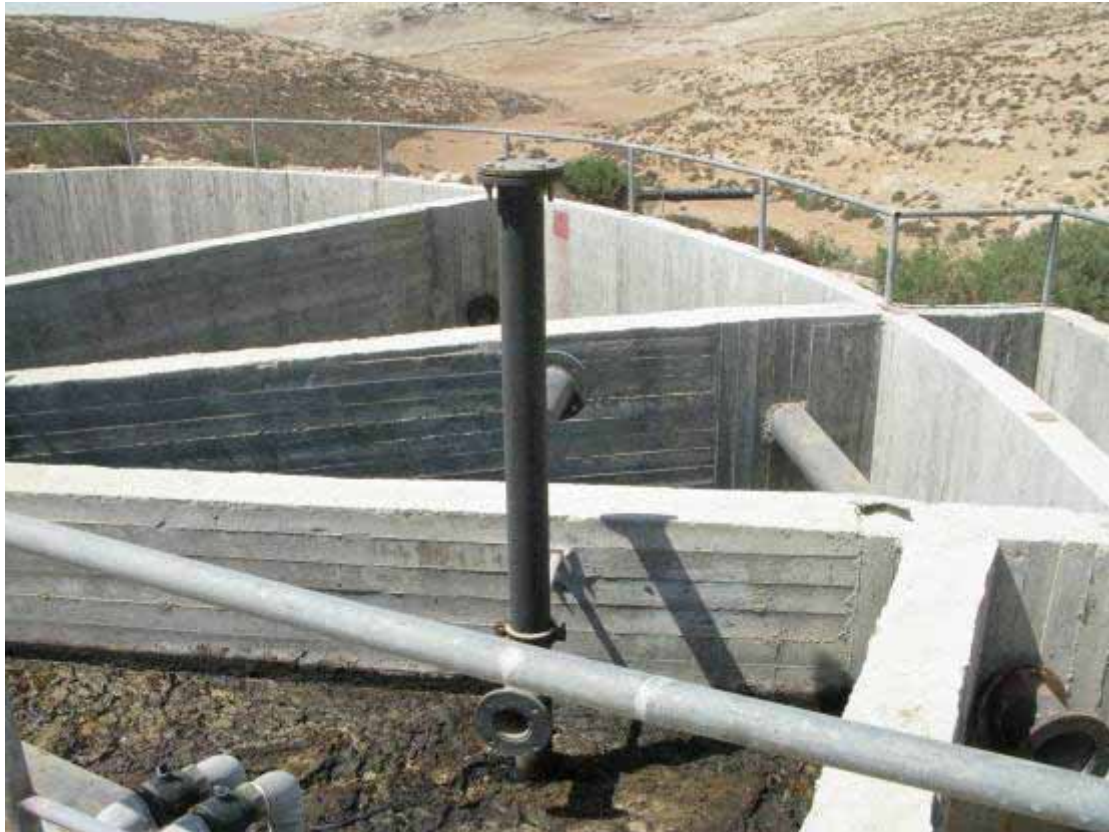
Out-of-order wastewater treatment facility in the Meitarim industrial area. Photo: Eyal Hareuveni, 15 Sept. '08.
