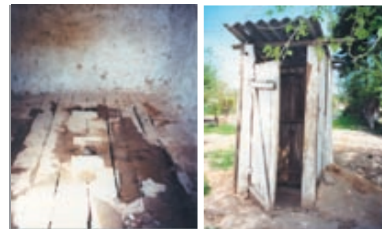
The condition of a school toilet in Central Asia
