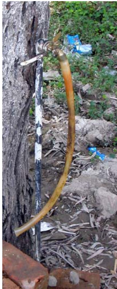
An illegal connection.
