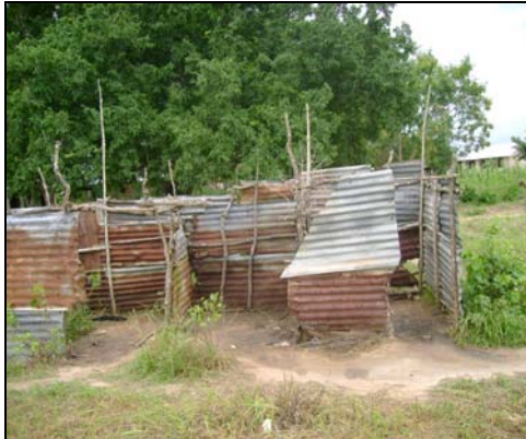
Plate 1: Existing structures in Nzovuni primary school which serves as latrine for girls (CRS K 2008)
