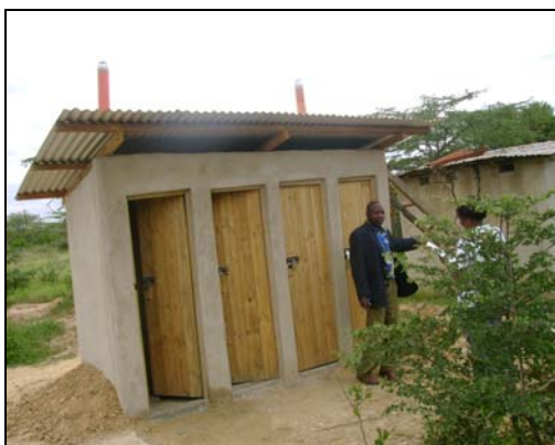
Plate 4: Mr. Kenga, the Head Teacher at Chapungu primary school reviews progress in the construction and drainage of this block of 4 latrines for boys in the school (CRS 2008)
