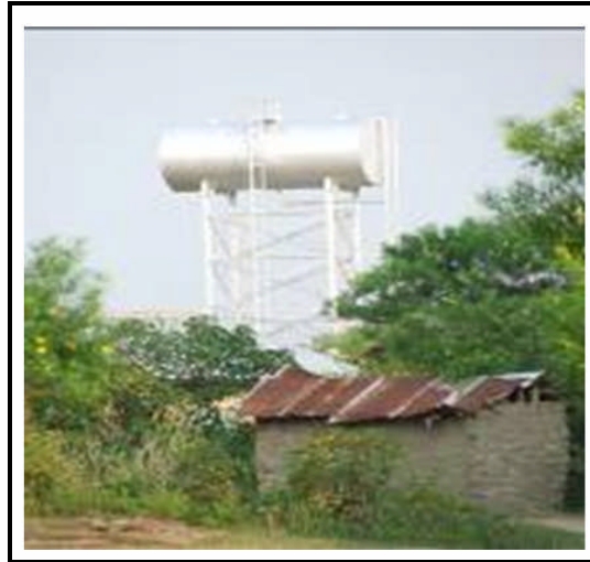
Figure 4-6: Tank of the piped water system in the RGC
