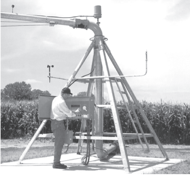
FIGURE 10.4 - The Central tower and the control panel.
