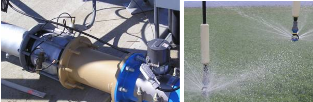
Figure 16. In-line pressure regulator (left) and individual pressure regulators (right)
