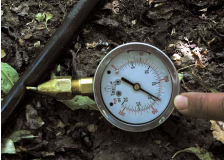
Figure 1. 30 psi pressure gauge with pitot tube stuck into tubing. Gauge is oil-filled.
