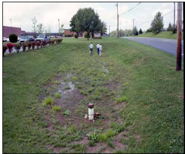
Figure 1: Surface Sand Filter
