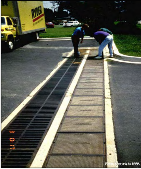
Figure 2: Sand filters are the preferred stormwater treatment option for hotspot retrofits.
