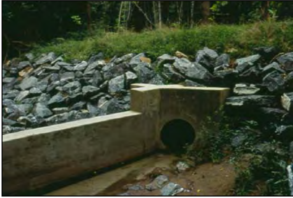
Figure 7: One technique for splitting flow from the conveyance channel for off-channel treatment.
