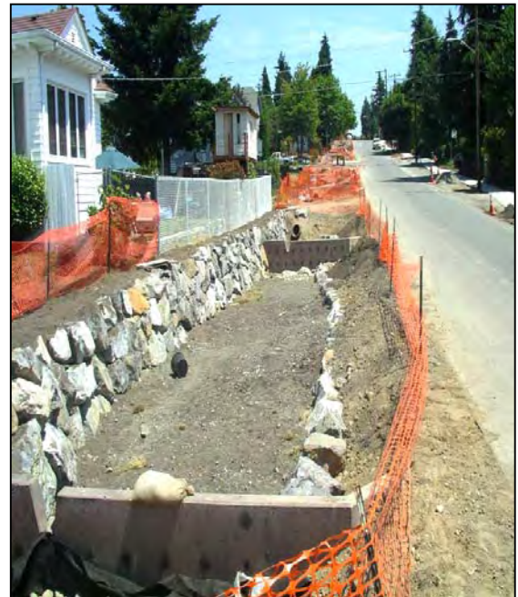
Figure 10: Construction sequencing is critical to maintain driveway access and minimize disruption to homeowners.
