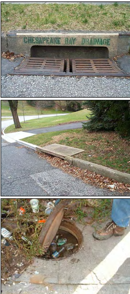
Figure 7: Crews check storm drains, grate inlets or manholes to determine depth of enclosed storm drainage.
