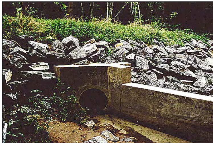
Figure 2: Parallel pipe inflow structure
