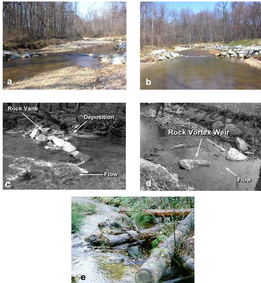
Figure 6: Other Stream repair practices that can promote baseflow channel creation include: (a) Double wing deflectors; (b) Rock cross vane; (c) Rock vane; (d) Rock vortex weir; and (e) Large woody debris
