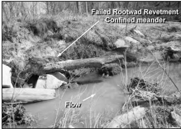
Figure 5: Failed rootwad revetment along a confined meander
