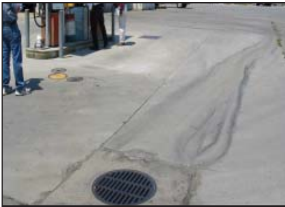
Figure 18: Stain from Uncovered Fueling Area Leading to Storm Drain
