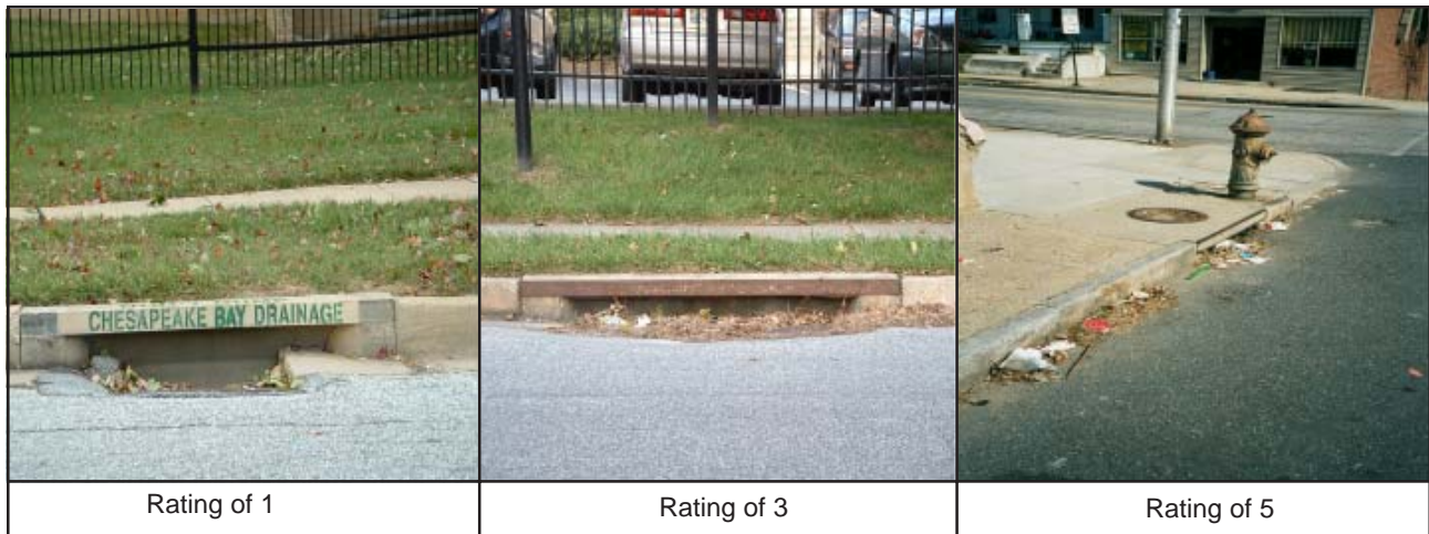
Figure 39: Varying Degrees of Trash and Debris Accumulation in Curb and Gutter and Storm Drain Inlets
