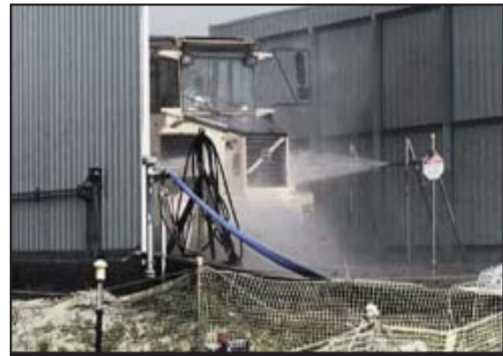
Figure 19: Dedicated Truck Wash Site with Runoff Controls
