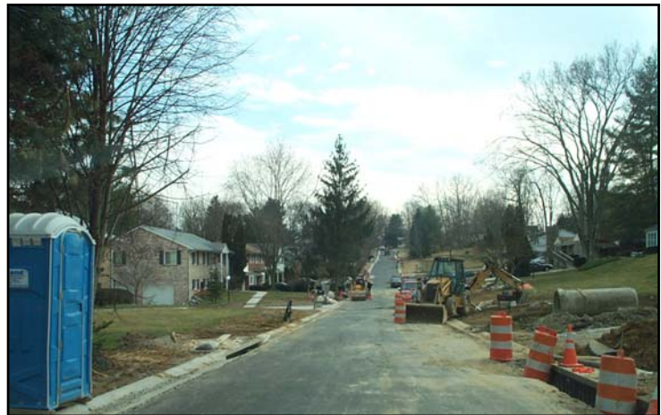
Figure 1: Roadway repairs and maintenance can generate significant amounts of sediment.
