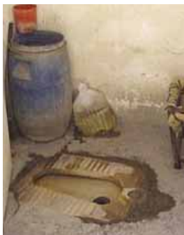
The latrine with no connection to a water faucet
