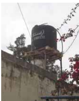
Cistern on the roof of an Arraneh house to store domestic water
