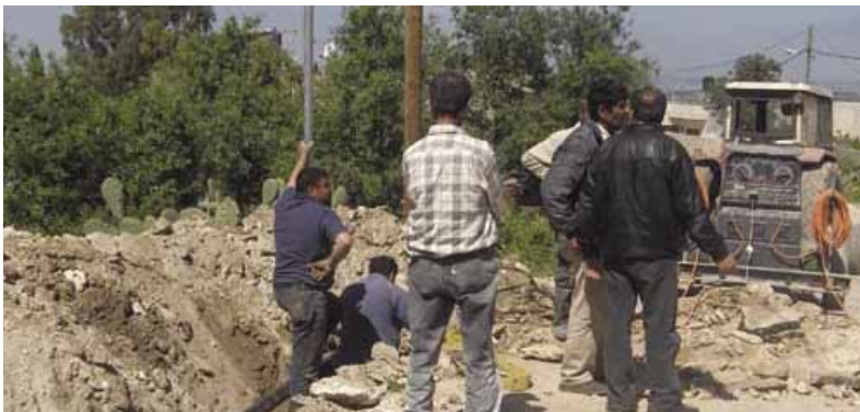
The new project to connect the water network to the high areas in Qabatya
