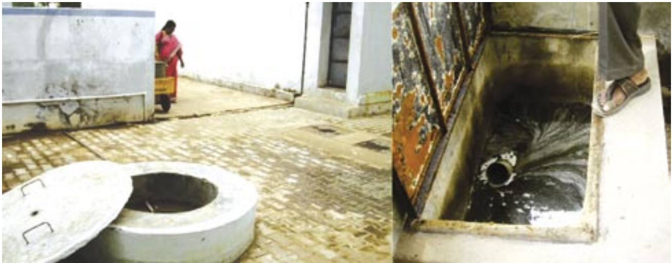
Biogas digester and outlet of gravel bed used in DEWATS
