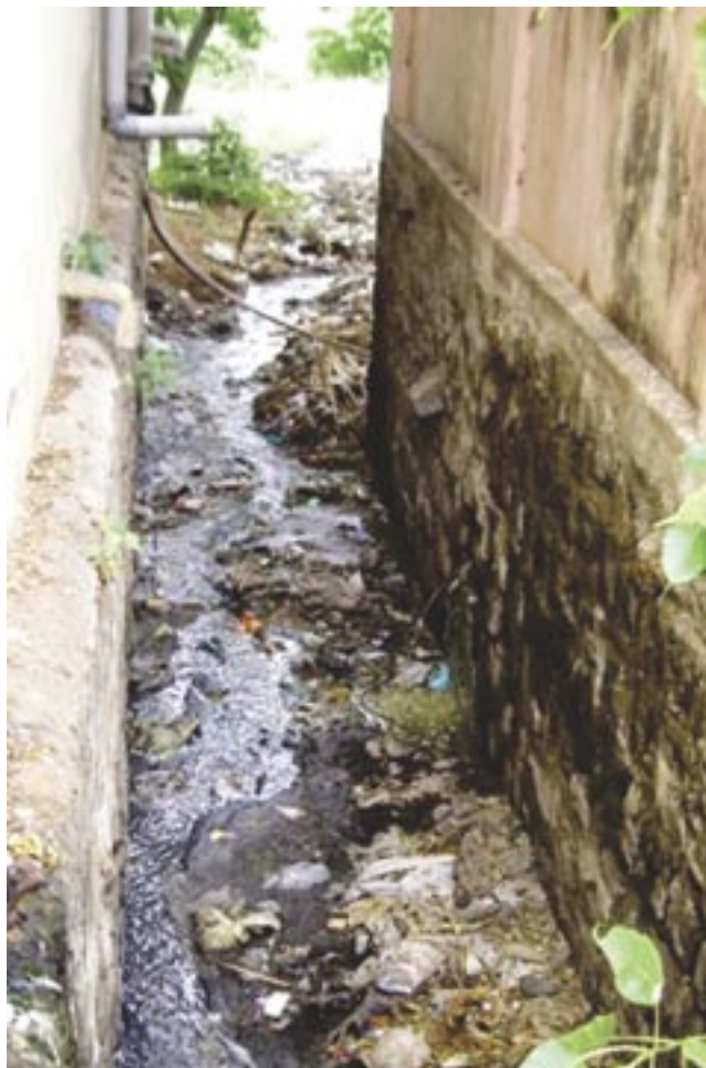
Leaking septic tank in Gorimedu
