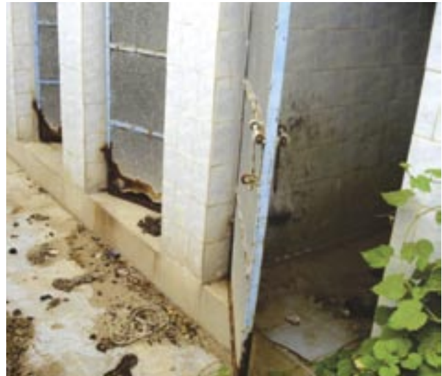
A new ISP in disrepair
