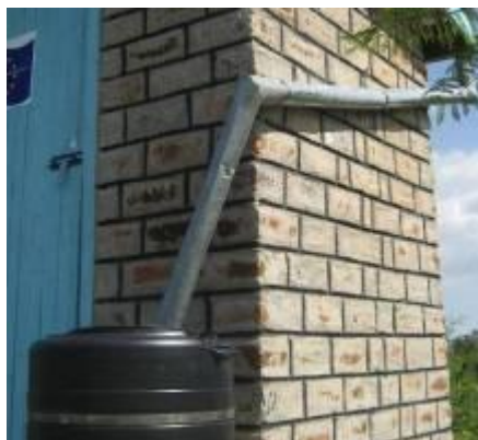
Down pipes fixed close to the wall to prevent children hanging on them
