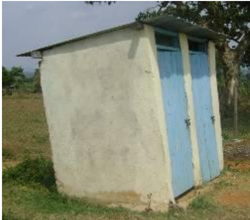
Collapsed simple pit latrine in Mumias
