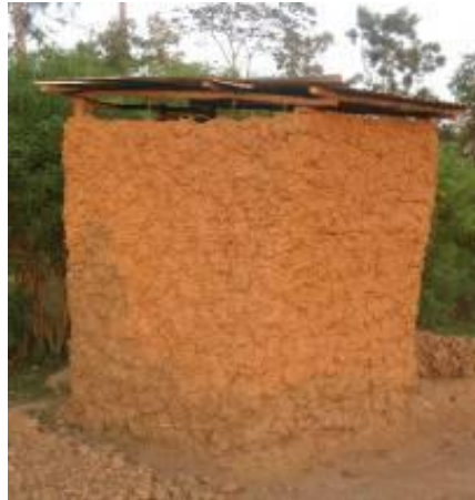
Simple local super structure from wooden sticks and earth (incl. earth plastering) in Ugunja
